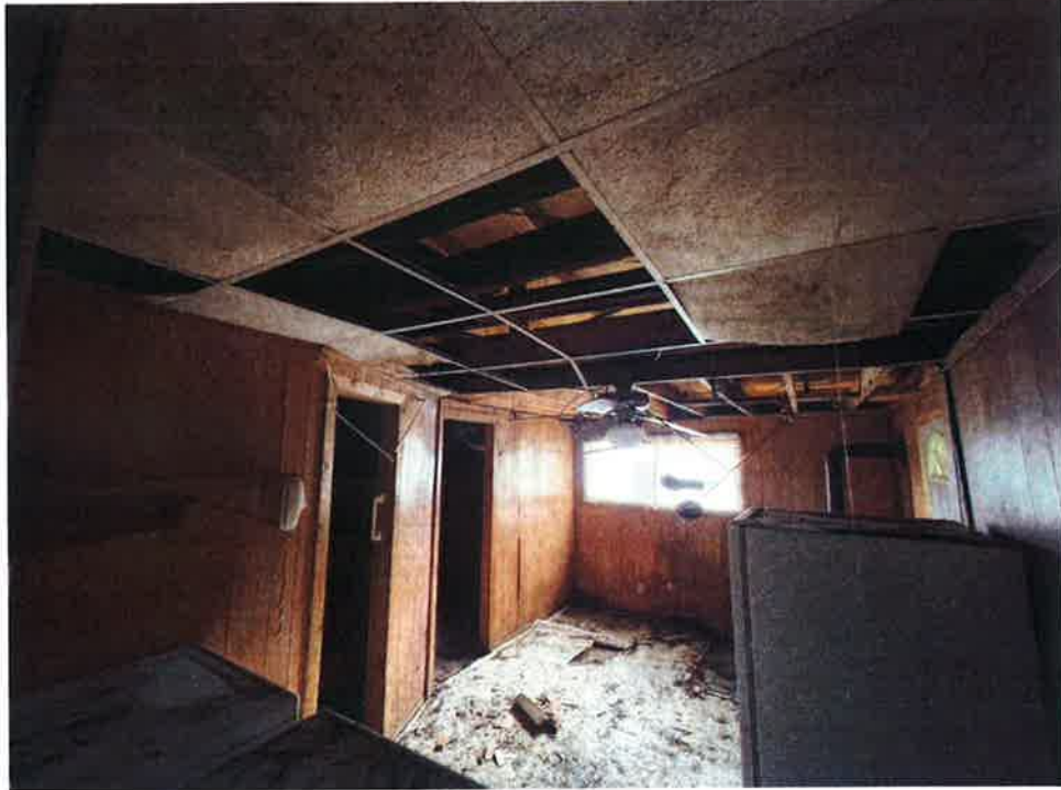
Wide view of 1F Laundry Room – missing SCT, debris on floor, delaminated flooring
