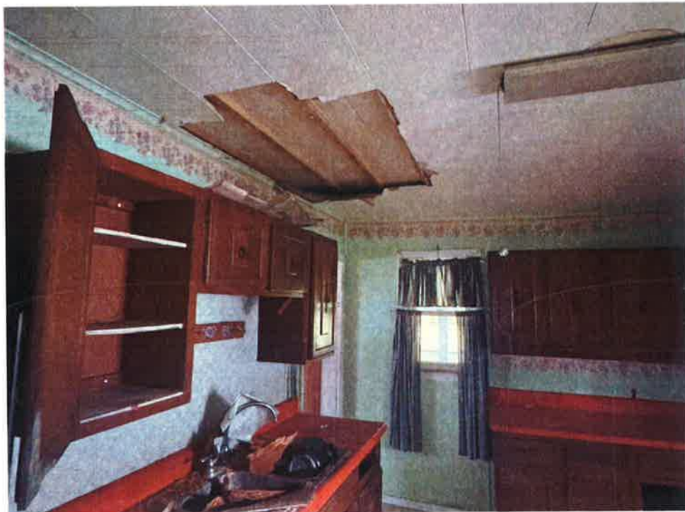
1F Kitchen Ceiling – missing damaged ceiling tiles
