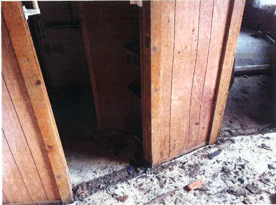
Water Damage debris on floor, and mold growth on wood paneling
