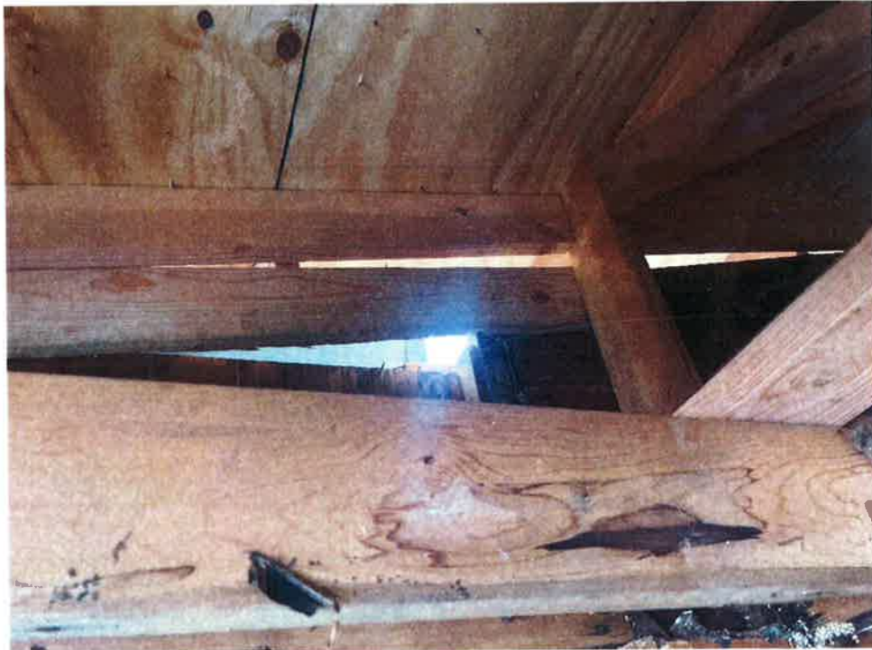
1F Laundry Room @ Ceiling – New Roof Base installed – visible light indicating opening to outside
