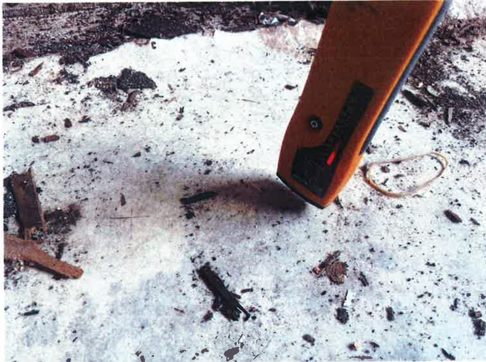
30% WME reading at Floor of 1F Laundry Room
