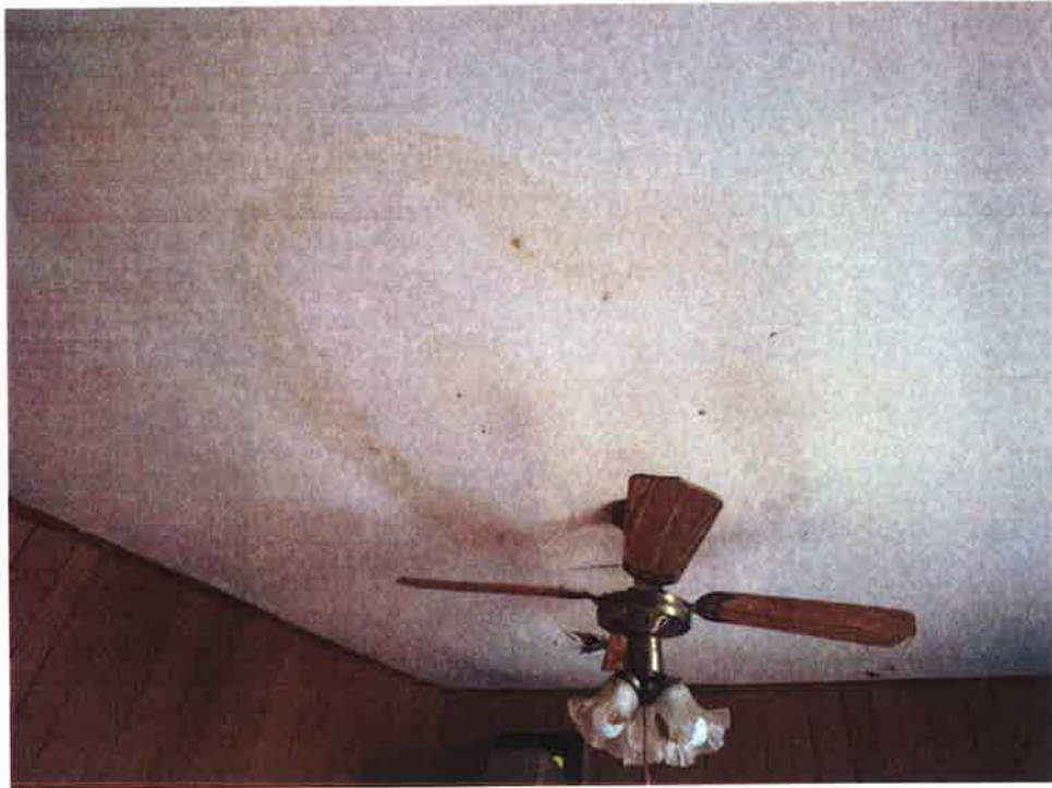
Water staining at ceiling in 1F Bedroom
