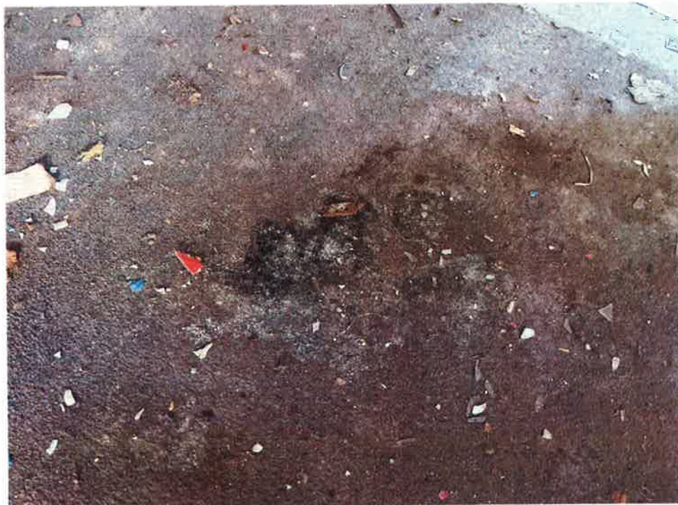
1F Living Room – Nasty spot at carpet flooring – verified to be a plethora of mold
