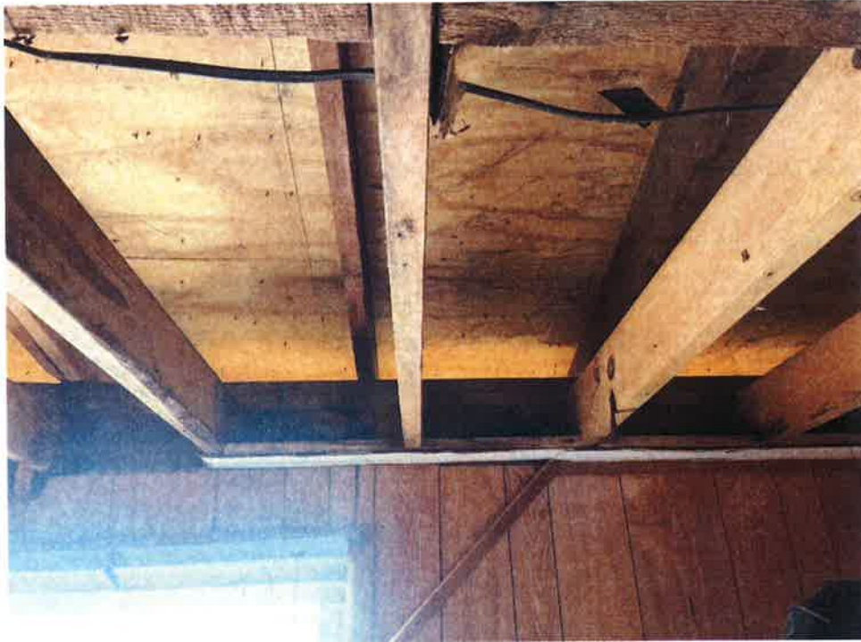
1F Laundry Room @ Ceiling – New Roof Base installed – visible light indicating opening to outside
