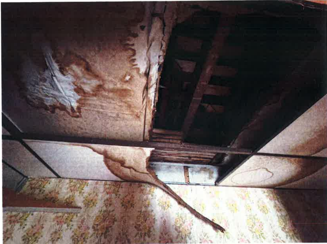
2F Front Bedroom East Closet – water staining with damage on old plaster & suspended ceiling
