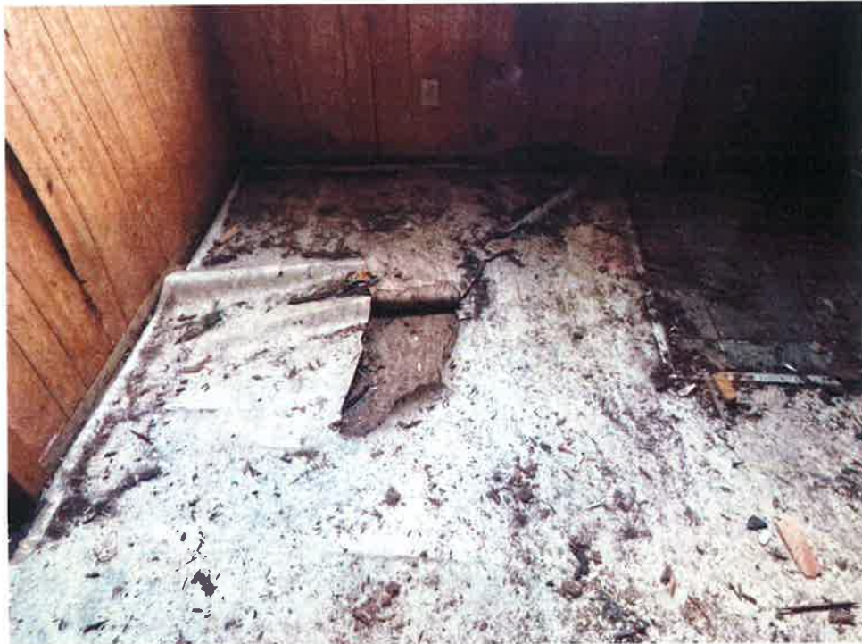
Delaminating Linoleum Floor in 1F Laundry Room
