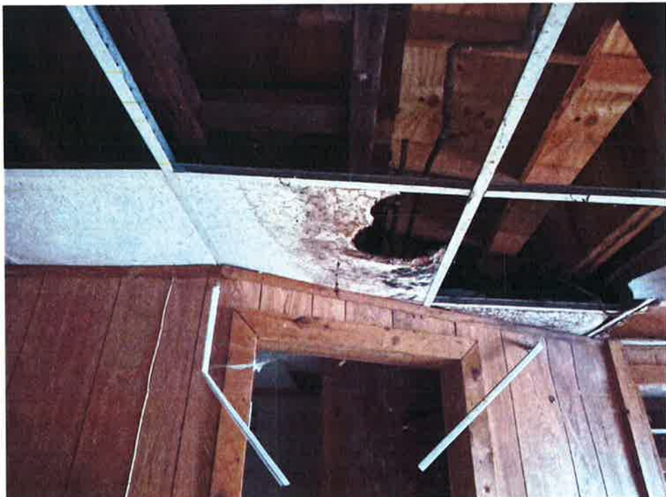
Missing/damaged Suspended Ceiling system. Mold growth visible as well.
