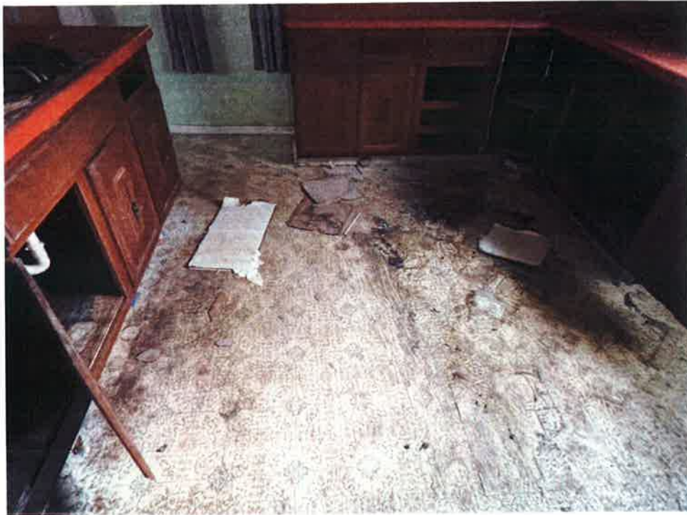
1F Kitchen – soiled linoleum flooring and fallen ceiling tiles
